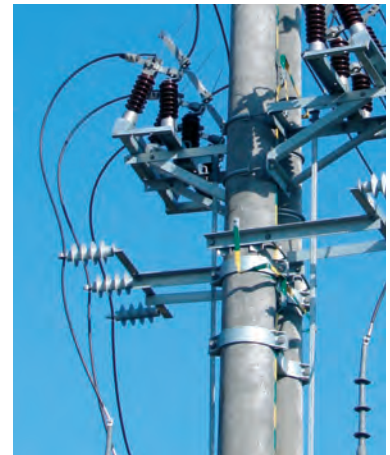
protection of MV cable – outlet of overhead line
